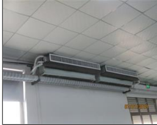
Photo of the inside of the main production hall Air conditioner in workshop.JPG
