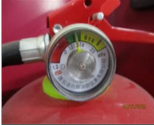
Photo of fire safety equipment Fire extinguisher in proper pressure.JPG
